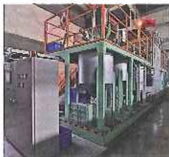
汚泥焼却灰からのりん回収装置 Equipment for phosphorus collection from sludge incineration ash
