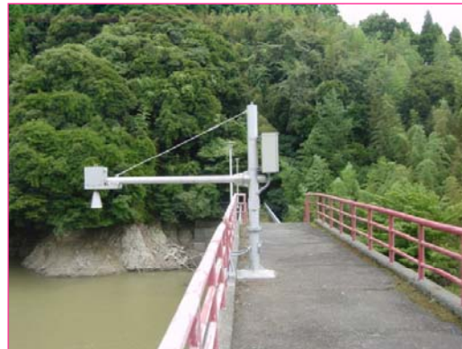
Irrigation dam control
