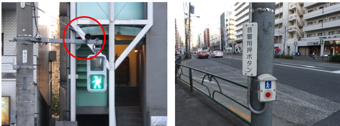
Figure 3.9 Example of Signal for Pedestrians (Left: Speaker, Right: Button for Visually Impaired Persons)
